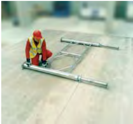
1. Connect ledger frame horizontally between 2 legs. Predetermined ledger frame position measured from headplate.
